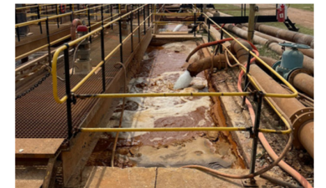
Figure 4: Untreated AMD water at Western Basin AMD Treatment Facility Settle Plant
